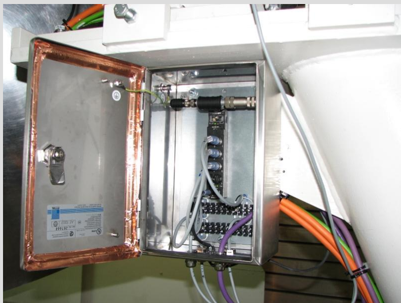
M3 Mirror Profibus Module inside shielded box
