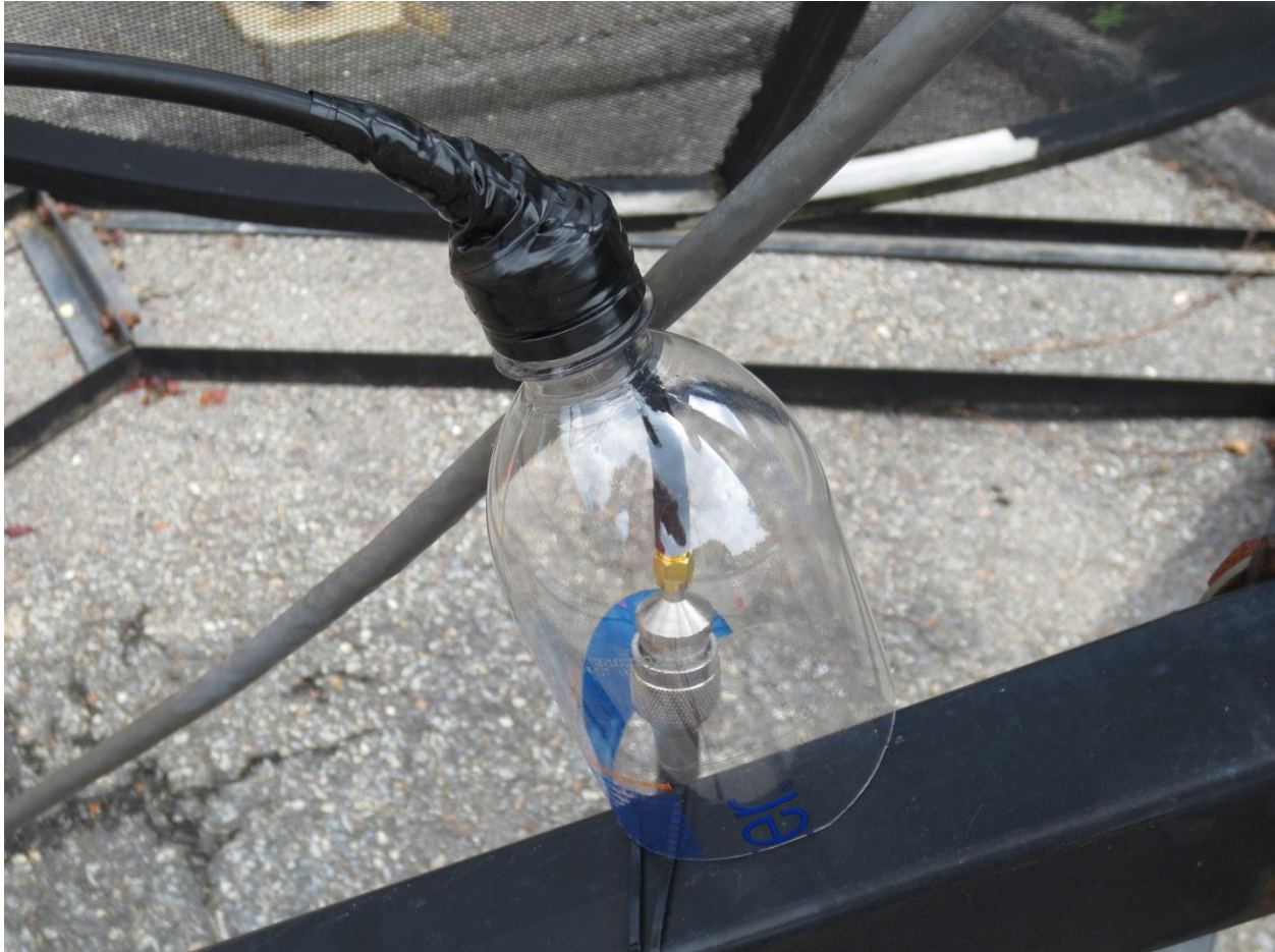
Figure 12: Weather-proof connection between the two coaxial cables.
